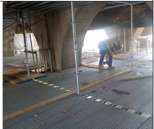
Ionion building containment on Level 2 in Pier 4 Bay 2 for 30-inch water main grinding
