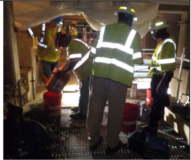
Test specimen sample for Fibrwrap placing Sika 211 concrete to deck pedestals Floor Beams 7-12
