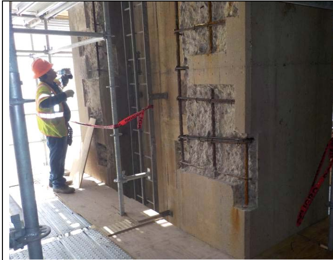
Fibrwrap installing rebar on Span D, N Elev, Rows EE-E, Level 4, Floor Beams 49-50
