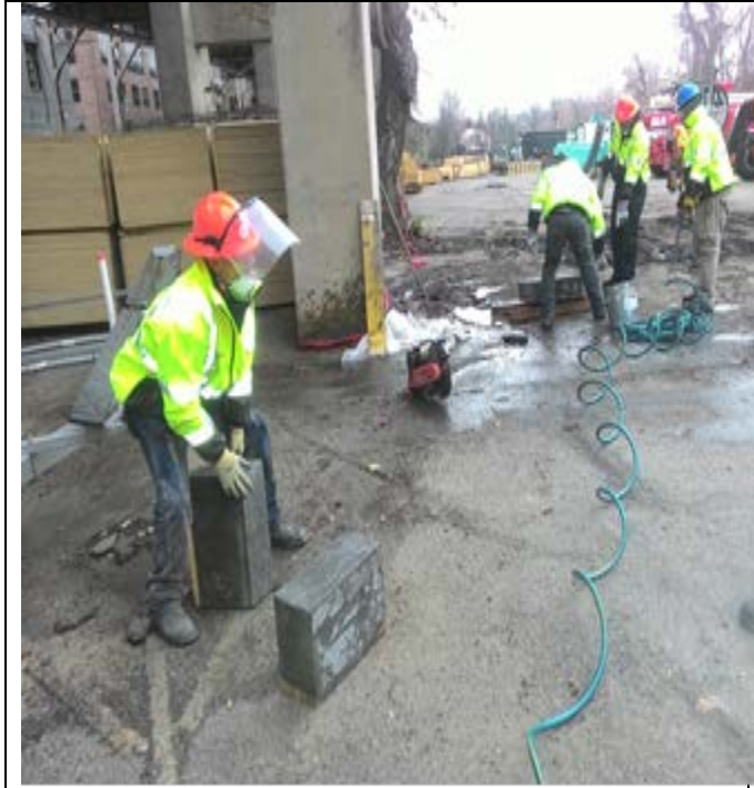
Fibrwrap strip Test Panel form with reinforcement to cut sectional for application
